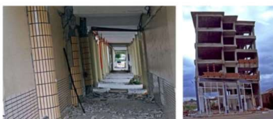
RC Structure (with conventional steel reinforcement) after earthquake excitation
